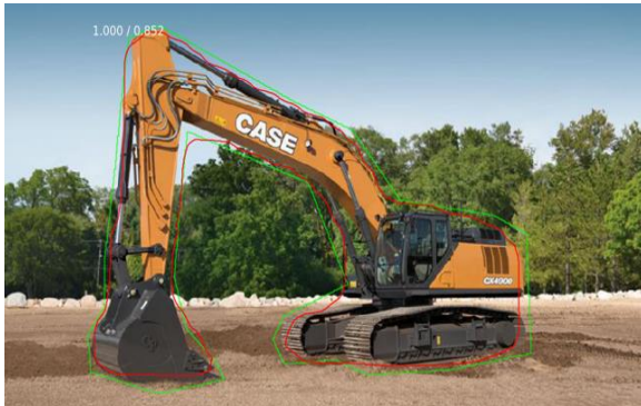
Figure 4. Excavator example (Confidence score/IoU), network prediction (red line) vs. ground truth (green line)
